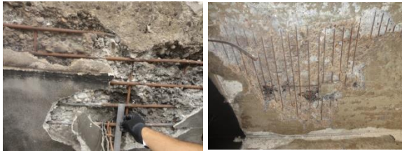
Fig. 3 Damaged concrete cover for slab reinforcements in the library hall.
