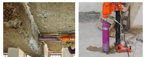
a) Core B at beam b) Core D at slab Fig. 10 Cores sampling.
