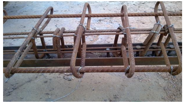
Plate 4: The steel reinforcing bar cage resting on the steel channel (with welded headed studs ) for a typical test beam .
