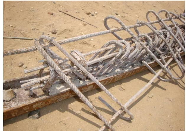
Plate 7: The steel channel and the attached headed studs of the damaged beam TB-U90 after removal of reinforced concrete , showing deformations of the studs .
