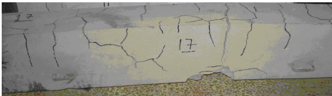
Figure (17) Crack pattern at failure for column C7 .
