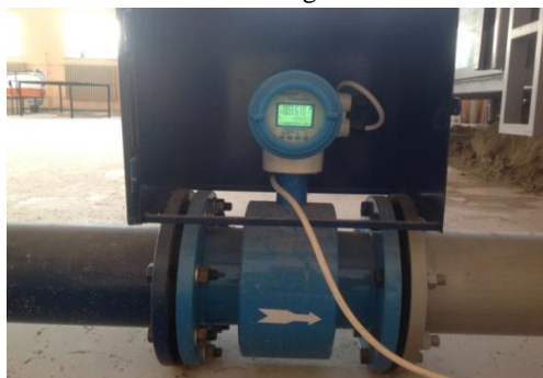
Fig. 2 Magnetic flow meter.
